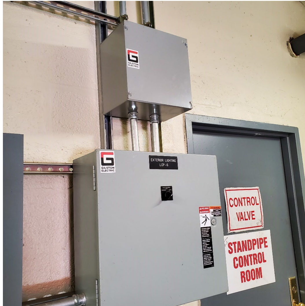
Exterior Lighting Controls
