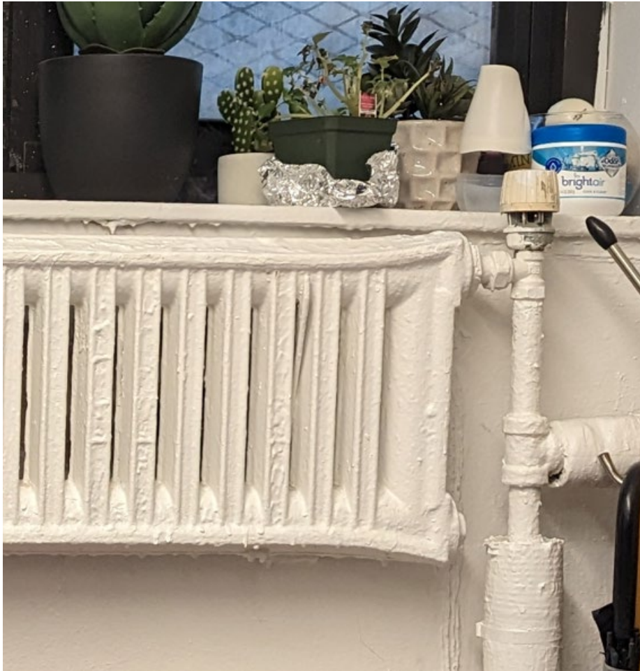
Two-pipe steam radiator with a TRV
