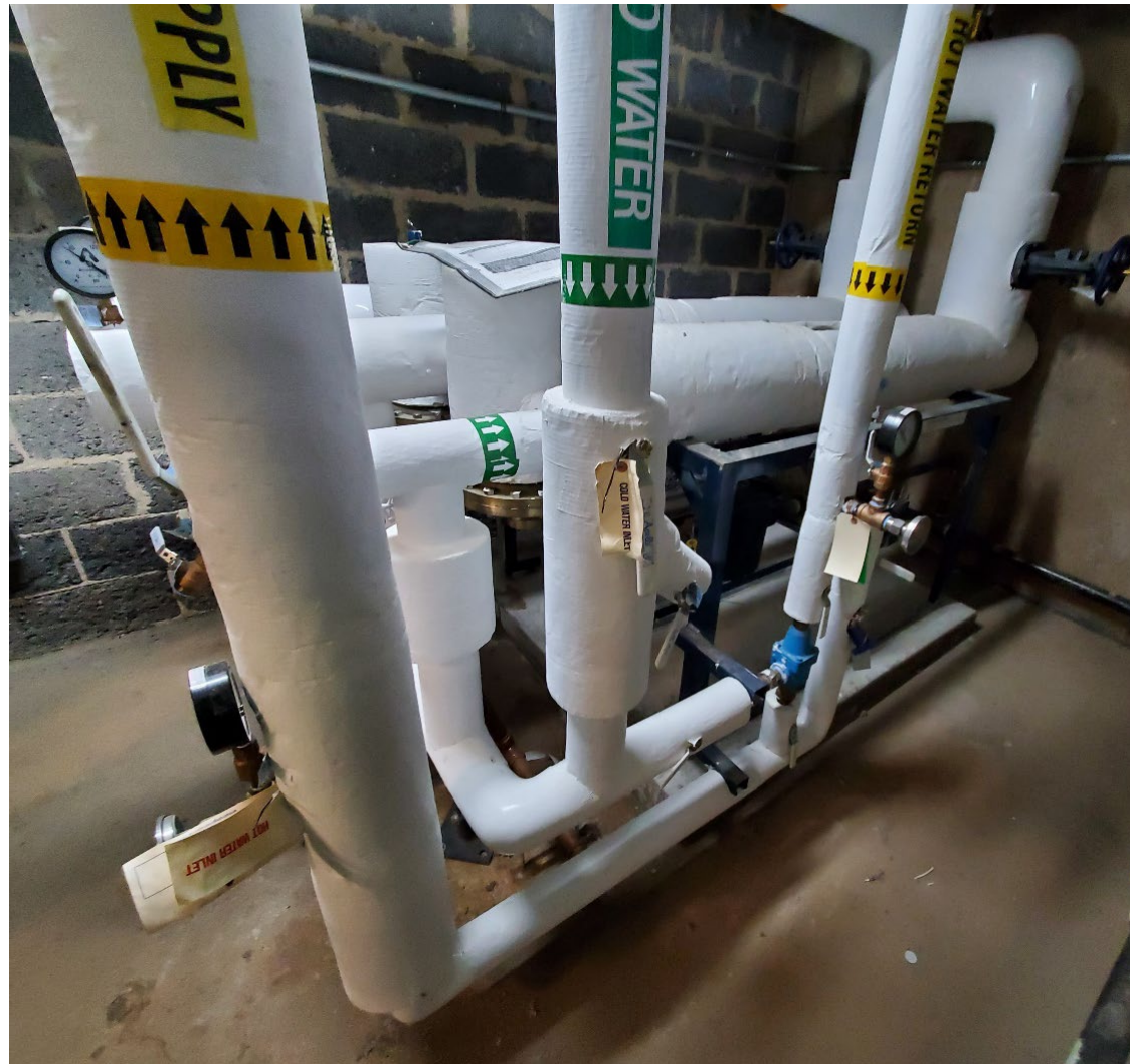
Insulated and labeled water pipes
