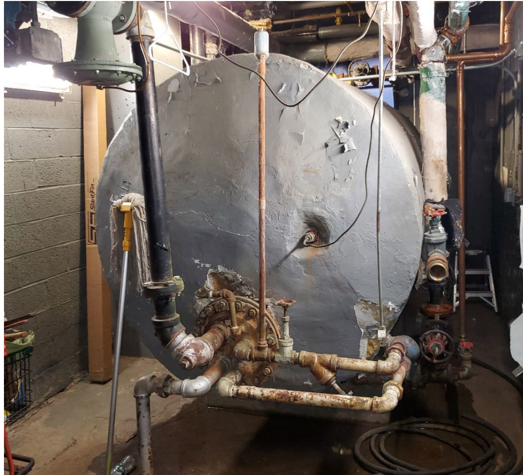
Insulated hot water tank
