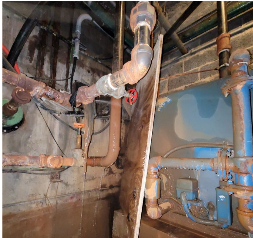
Water leak requiring repair
