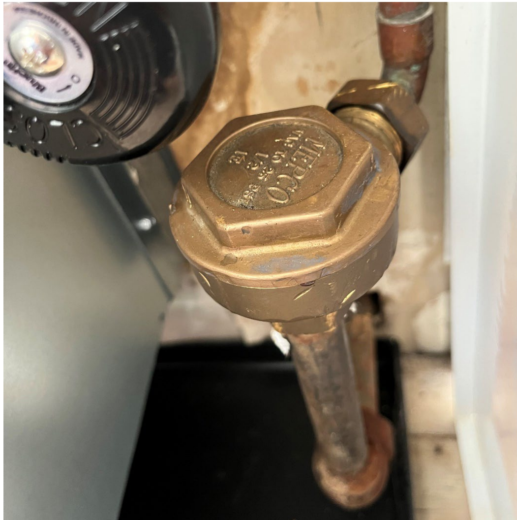
Thermostatic steam trap in a dwelling unit
