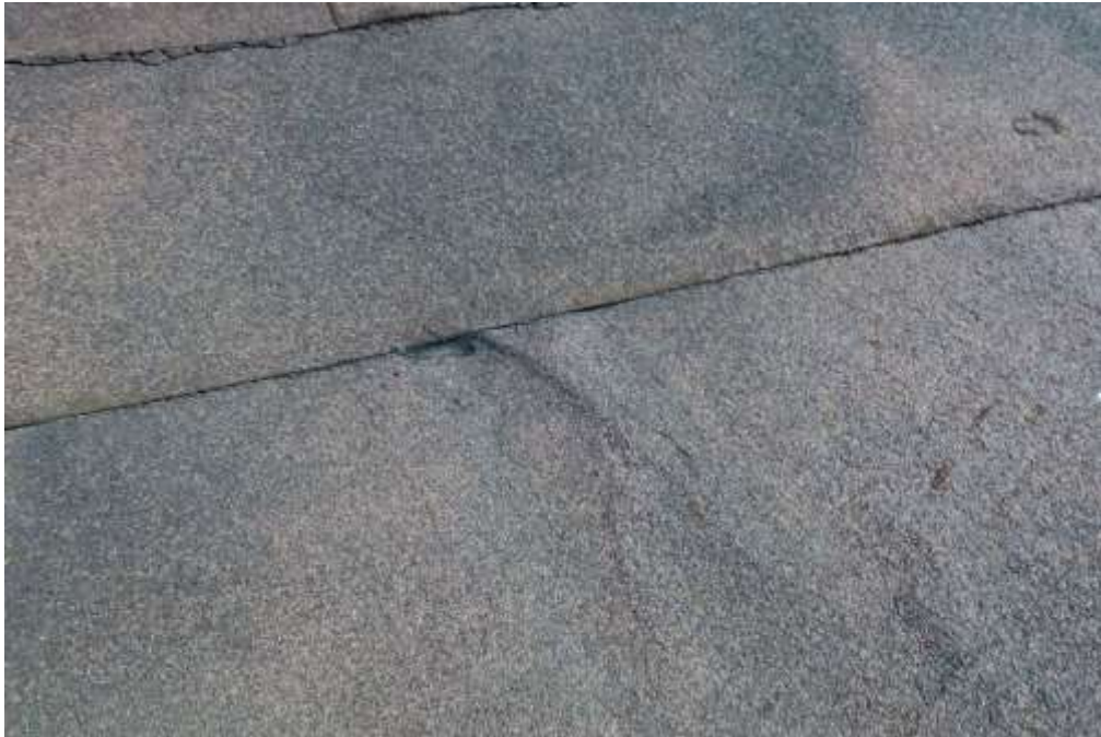
Roof blister with open seam
