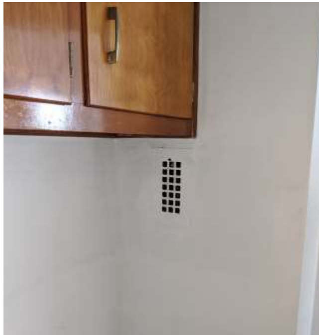
Kitchen Exhaust Grille
