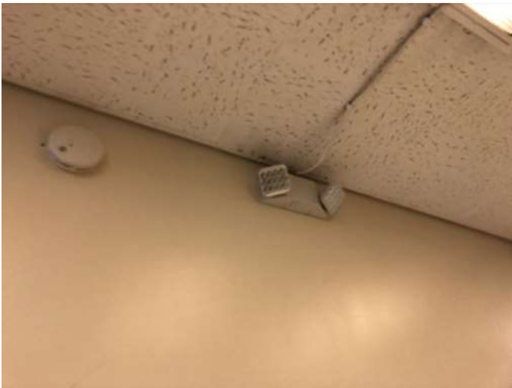
Typical Hallway Smoke Detector
