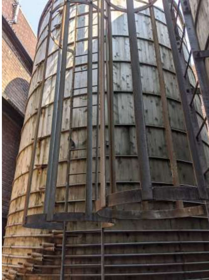
Main Domestic Water Tank
