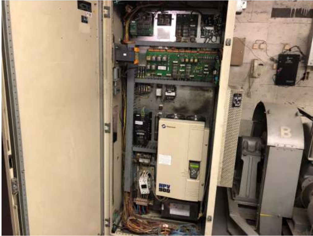
Typical Elevator Control Panel
