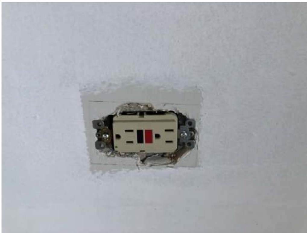
Typical Kitchen GFI Circuit Breaker
