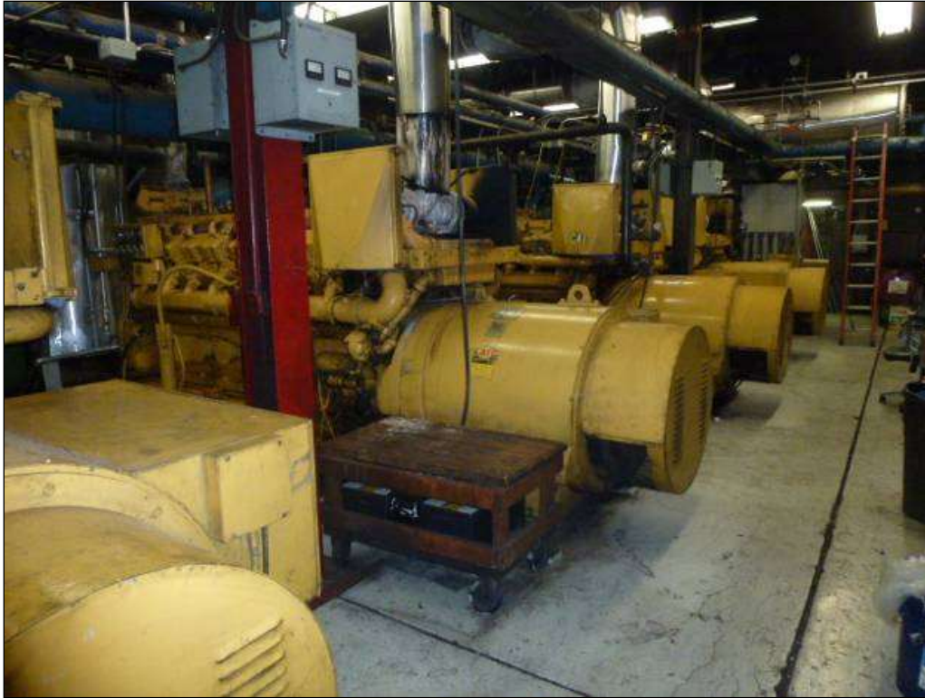
Power Plant Generators
