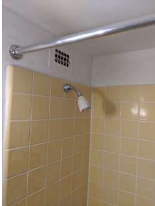
Typical Bathroom Exhaust Grille
