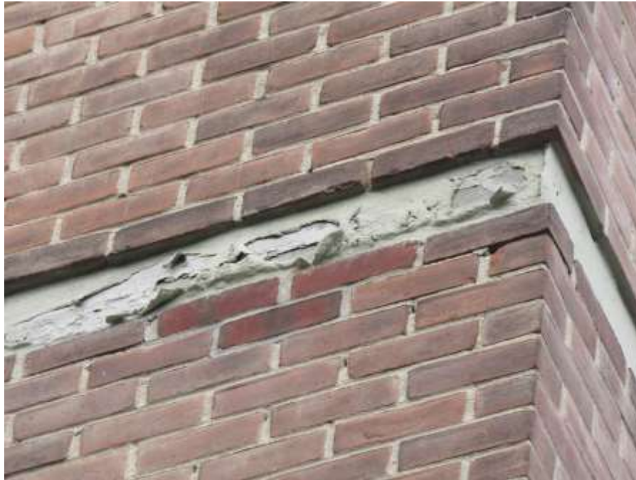
Peeling coating with spalled patching
