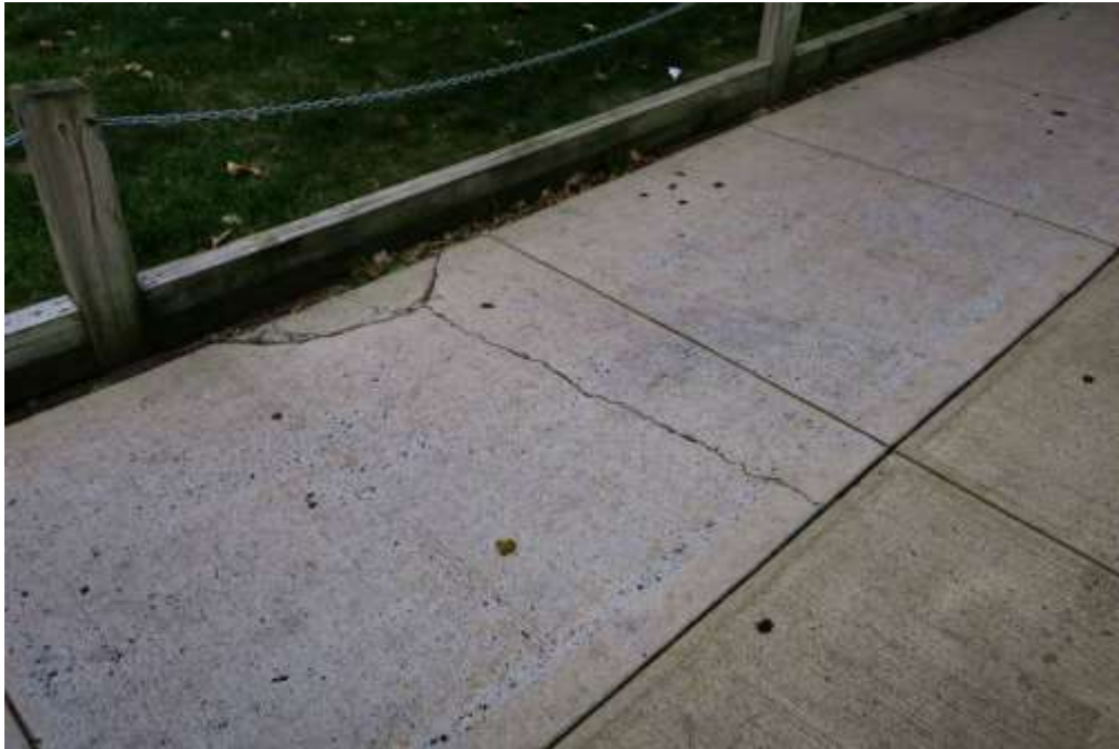
Cracked walkway flag
