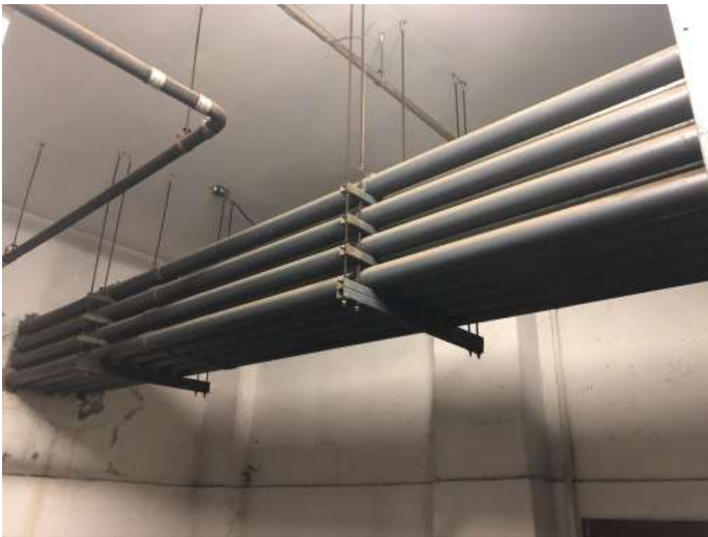
Supply Feeders From Power Plant
