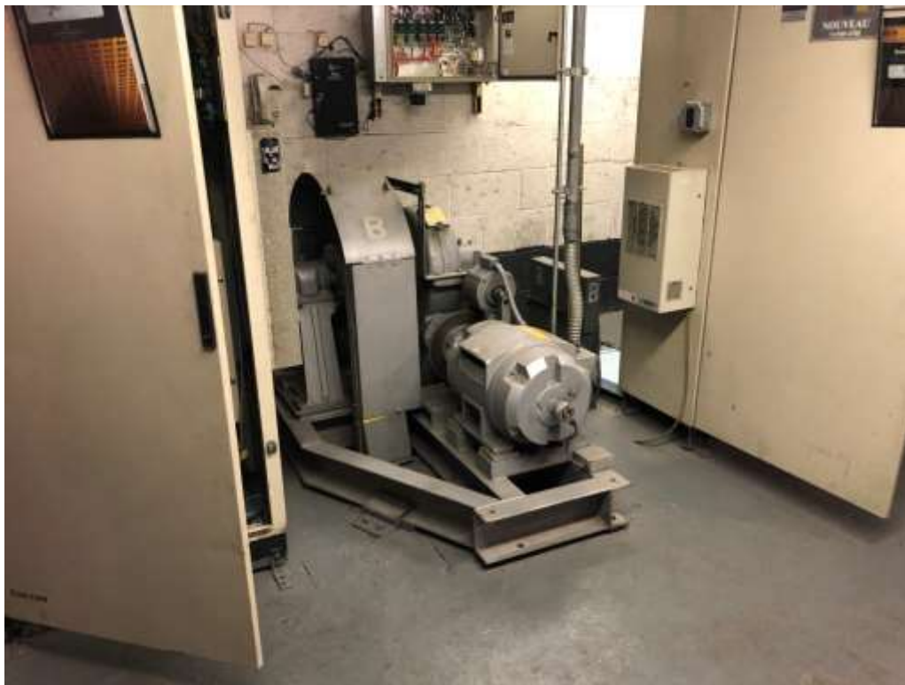
Typical Elevator Motor
