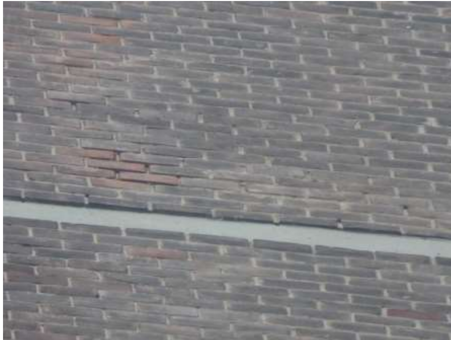
Open mortar joints
