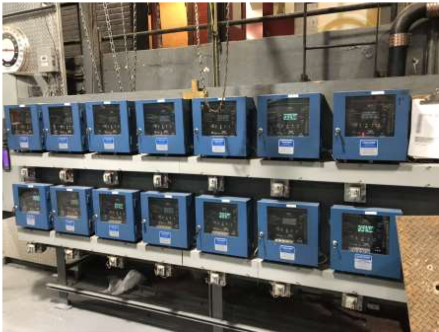
Heating System Control Panels
