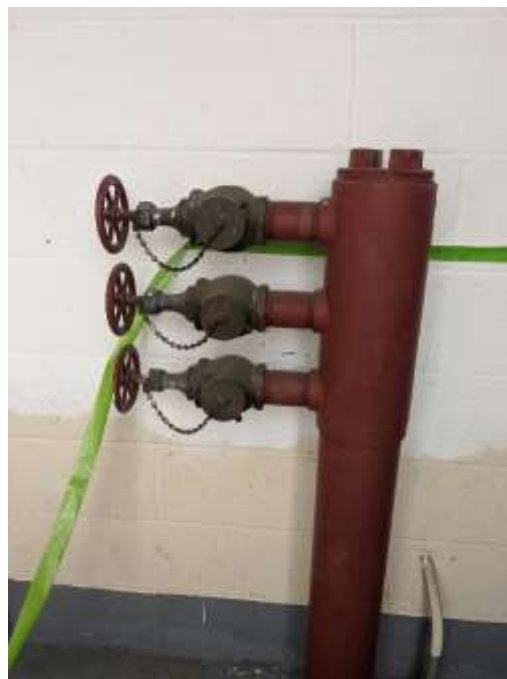
Typical Fire Standpipe Manifold at Roof
