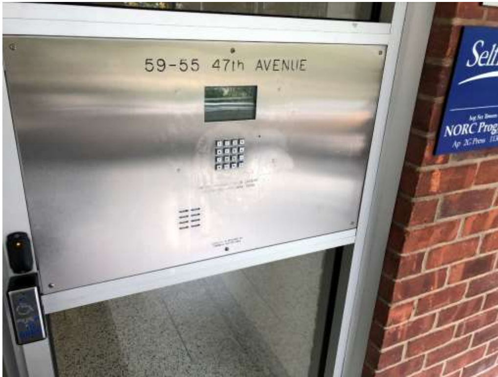
Intercom System – Wireless Based
