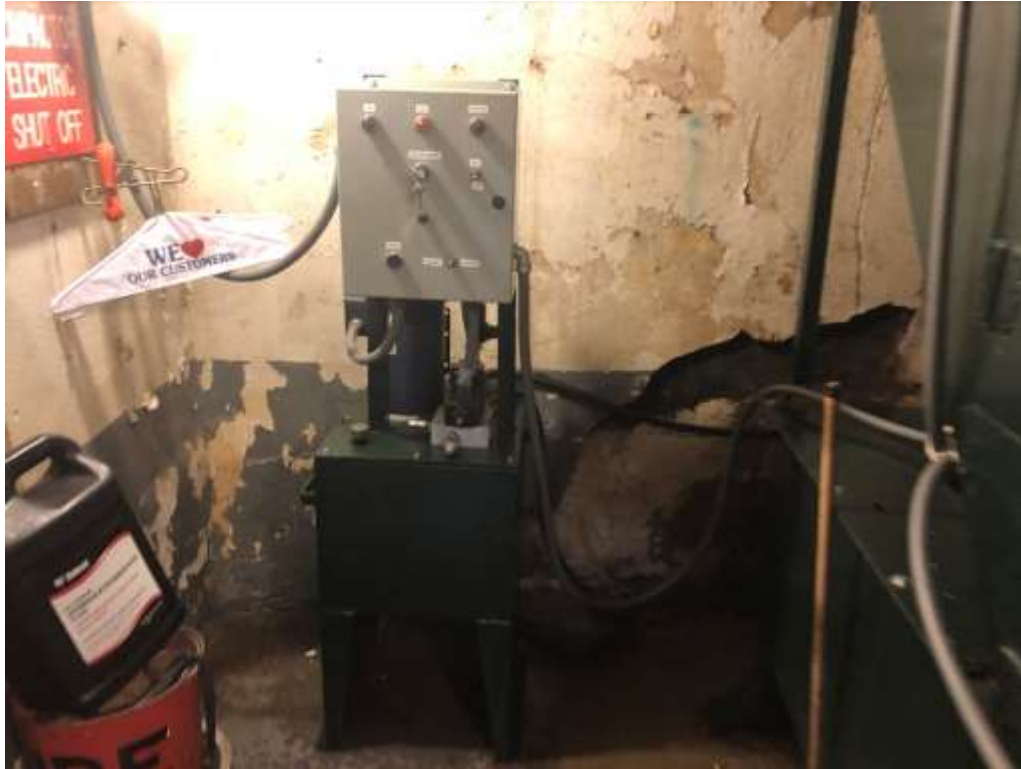
Typical Compactor Compressor
