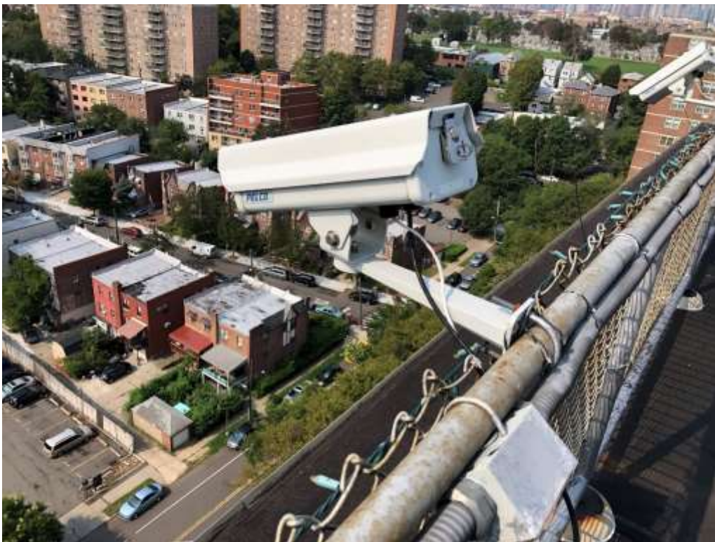
Typical Exterior Camera
