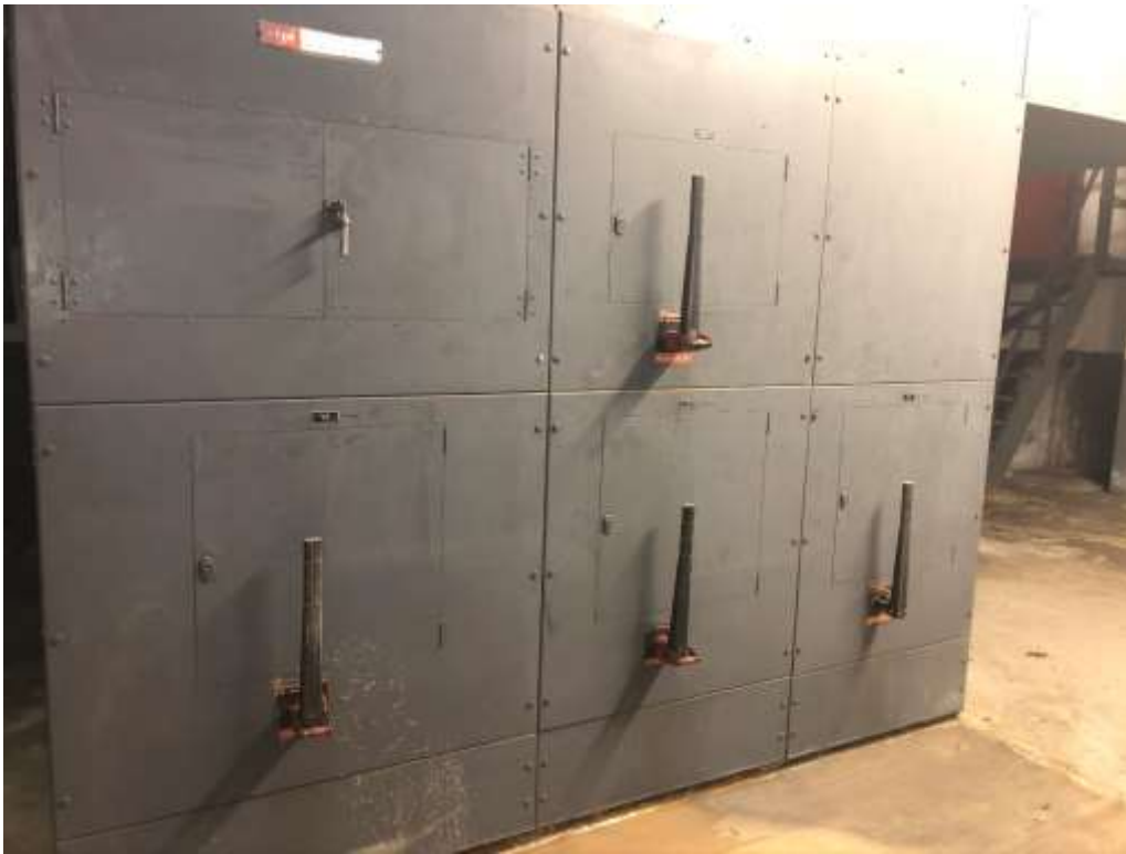
Buildings' Main Distribution Panel Section 1
