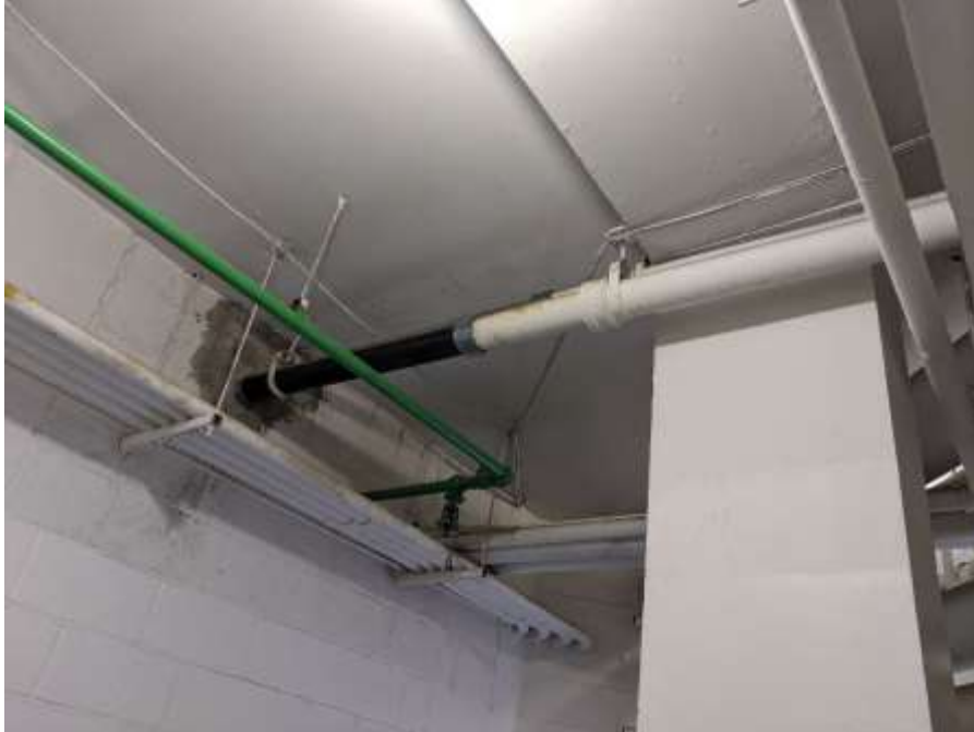
Typical Sanitary Waste Line with replaced portion
