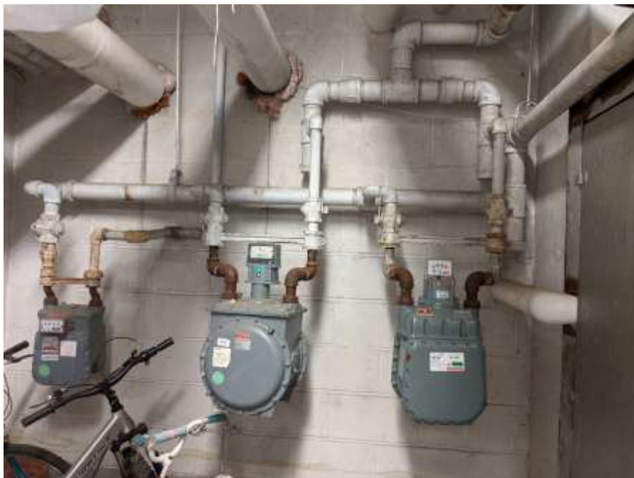
Typical Gas Meters
