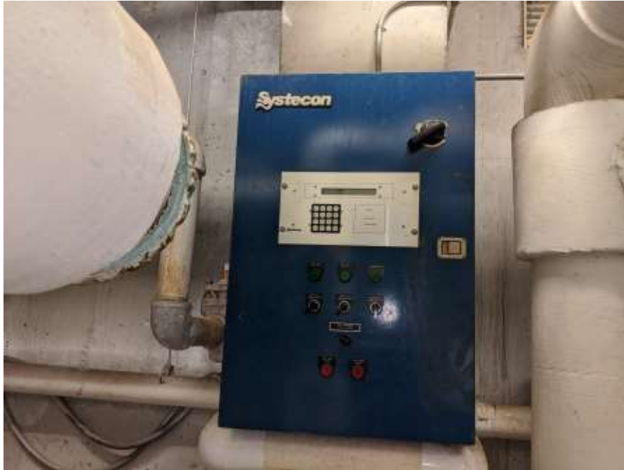
House Pump Control Panel
