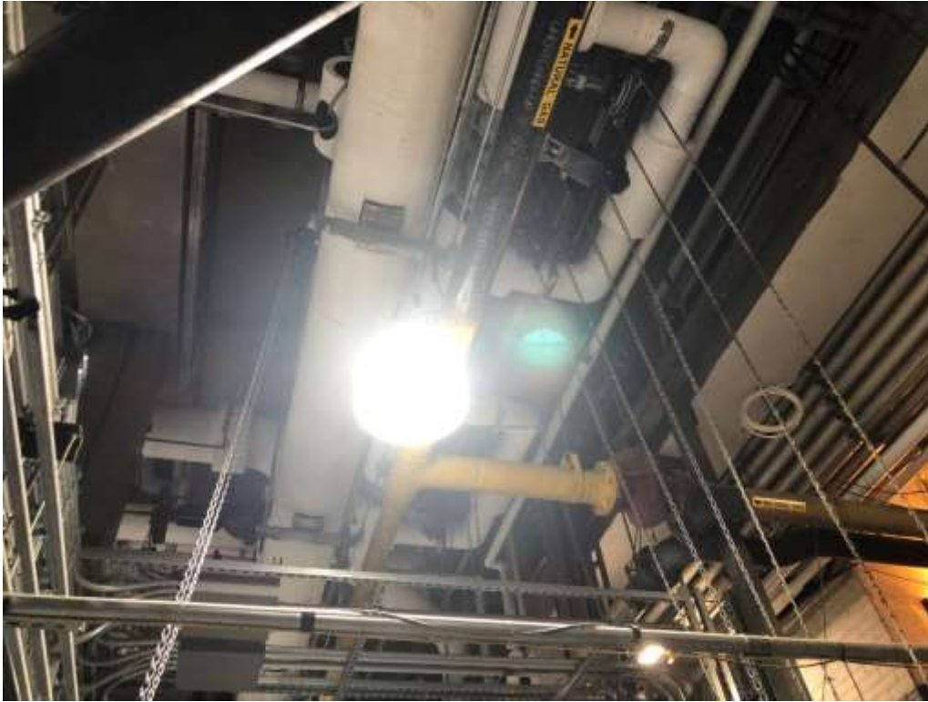
Boiler Room High-Hat LED Lighting Fixture
