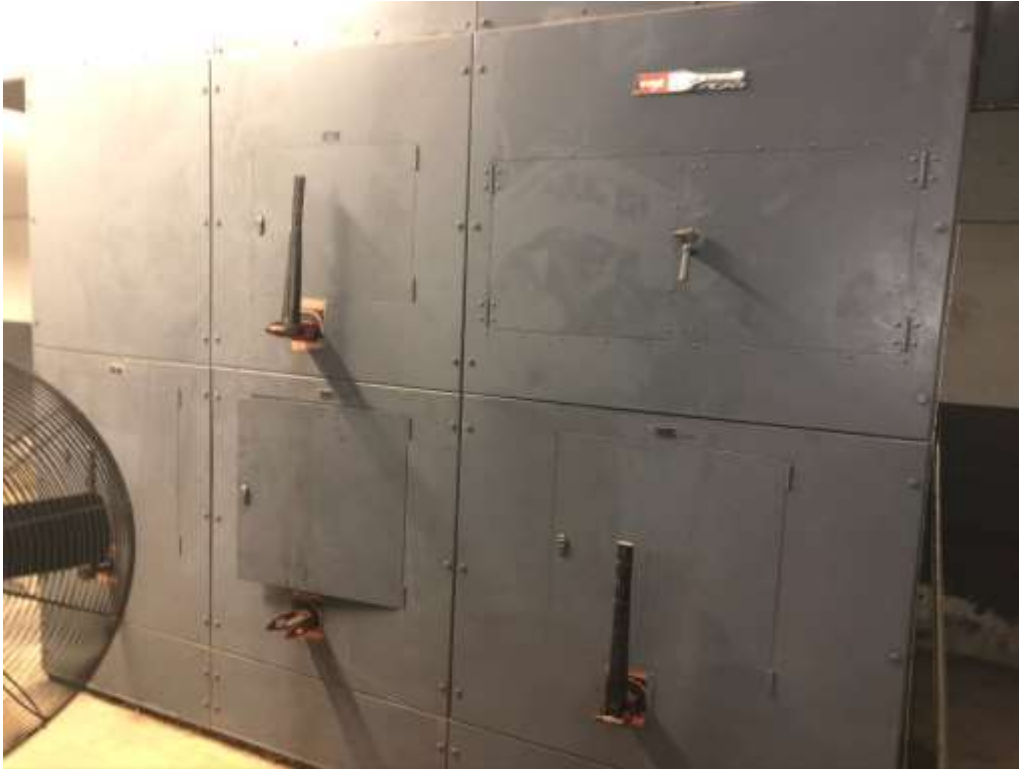
Buildings' Main Distribution Panel Section 2
