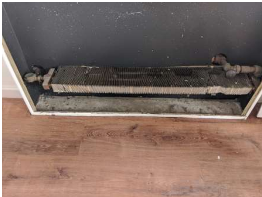
Typical Apartment Heating Convactor with Manual Shut-off Valve & Steam Trap
