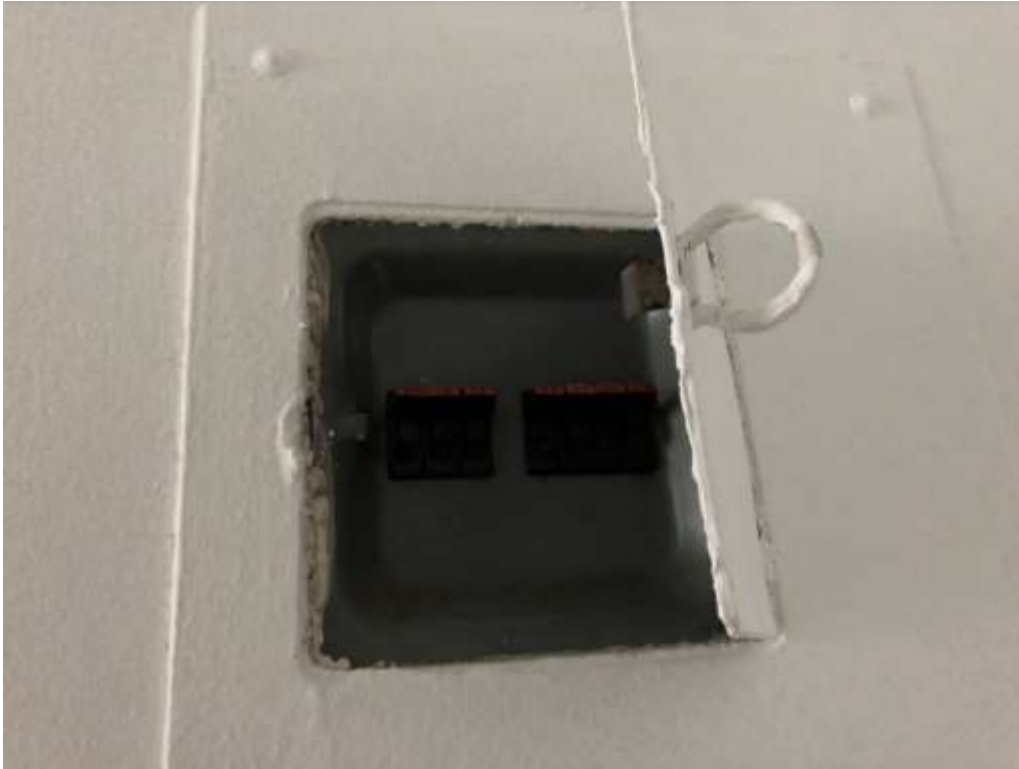
Typical Federal Pacific Circuit Breaker Panel
