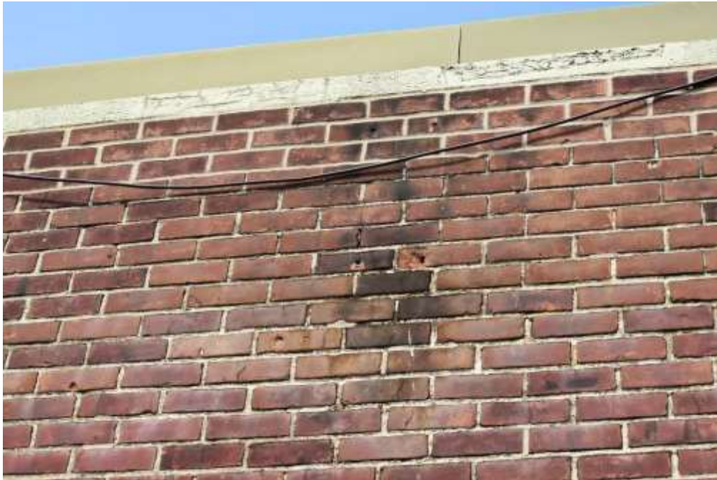
Open mortar joints and spalled brick at bulkhead
