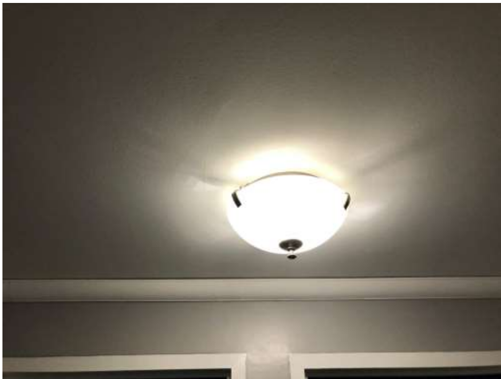
Typical Hallway Lighting Fixture
