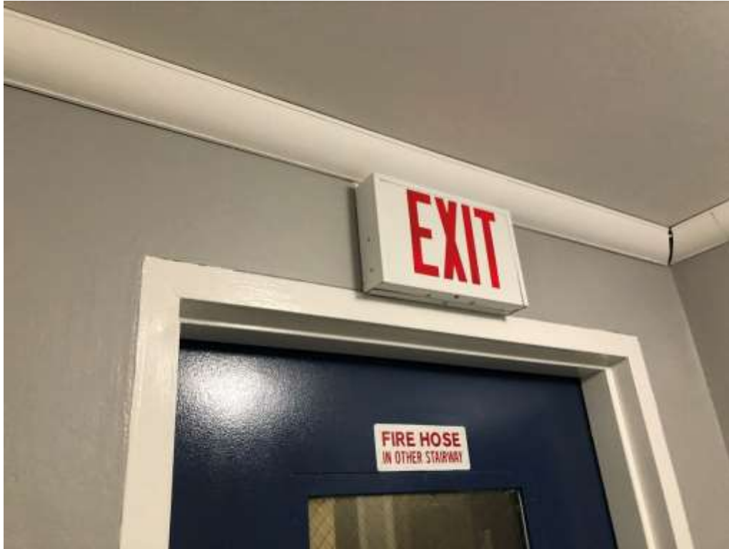
Typical LED Exit Sign – Hallway
