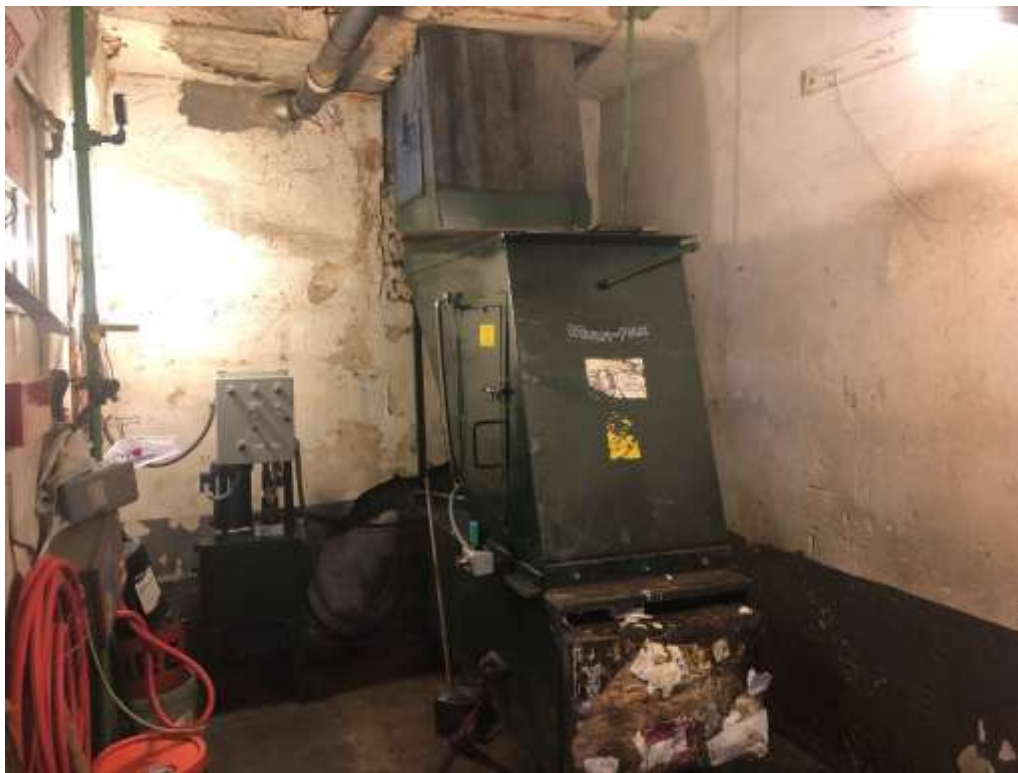
Typical Compactor Machine – No Name Plate
