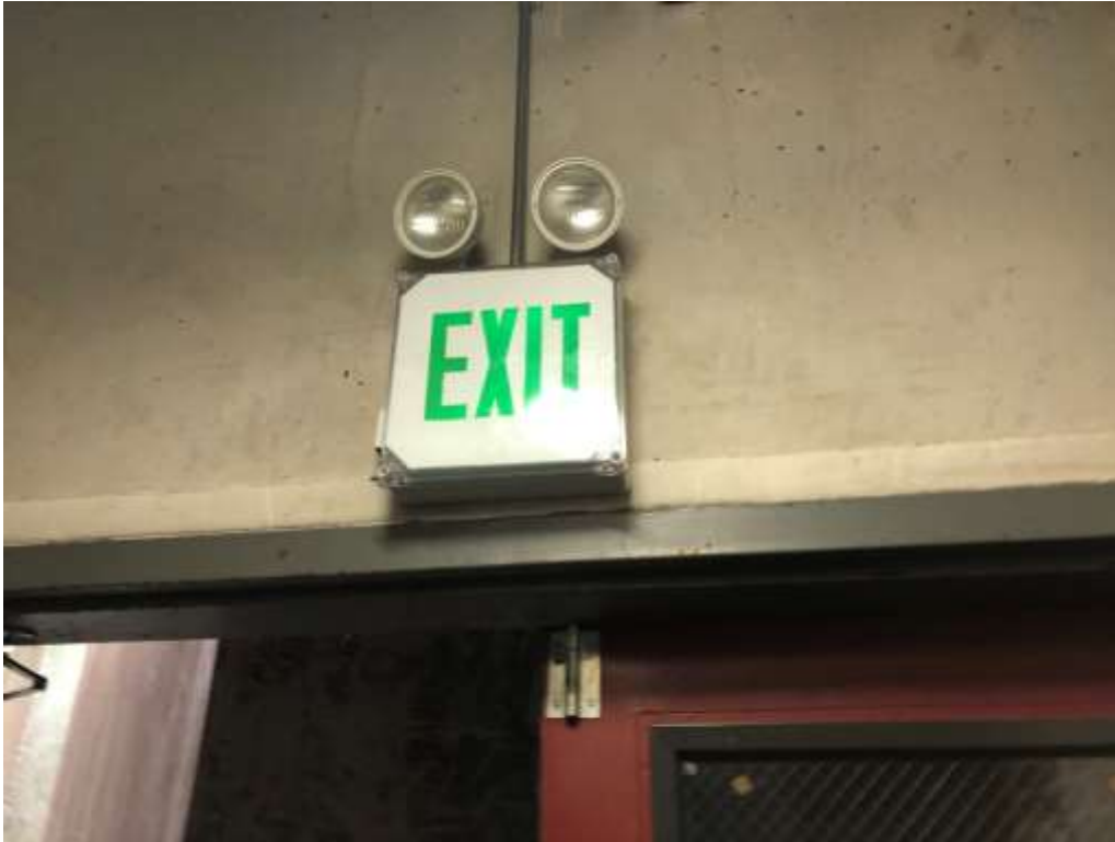
Typical LED Exit Sign – Common Areas
