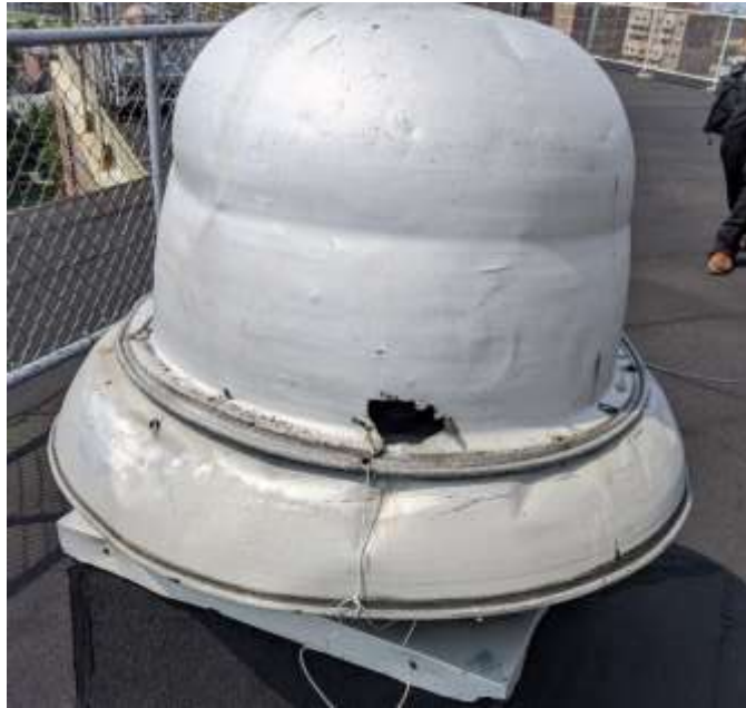
Typical Roof Exhaust Fan Original – Roof
