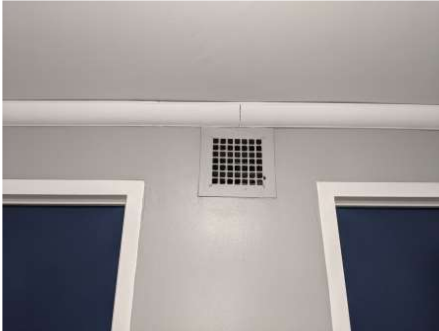
Typical Hallway Exhaust Grille
