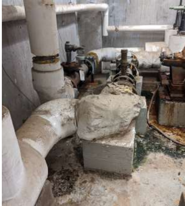
Domestic Water Services with Water Meters
