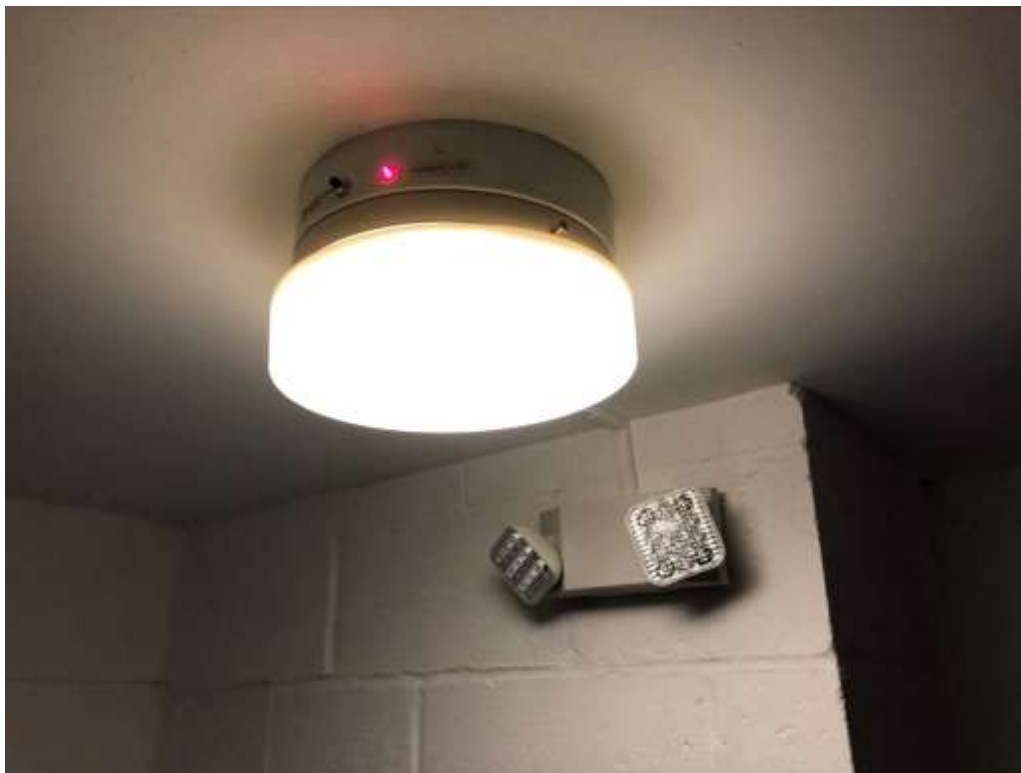
Typical Stairwell Lighting Fixture with Battery Backup
