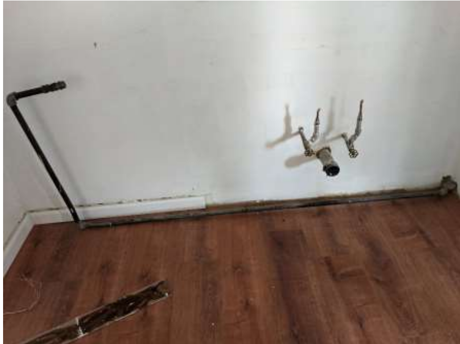
Typical Plumbing Piping (Gas, water, and Sanitary Waste) in Kitchen
