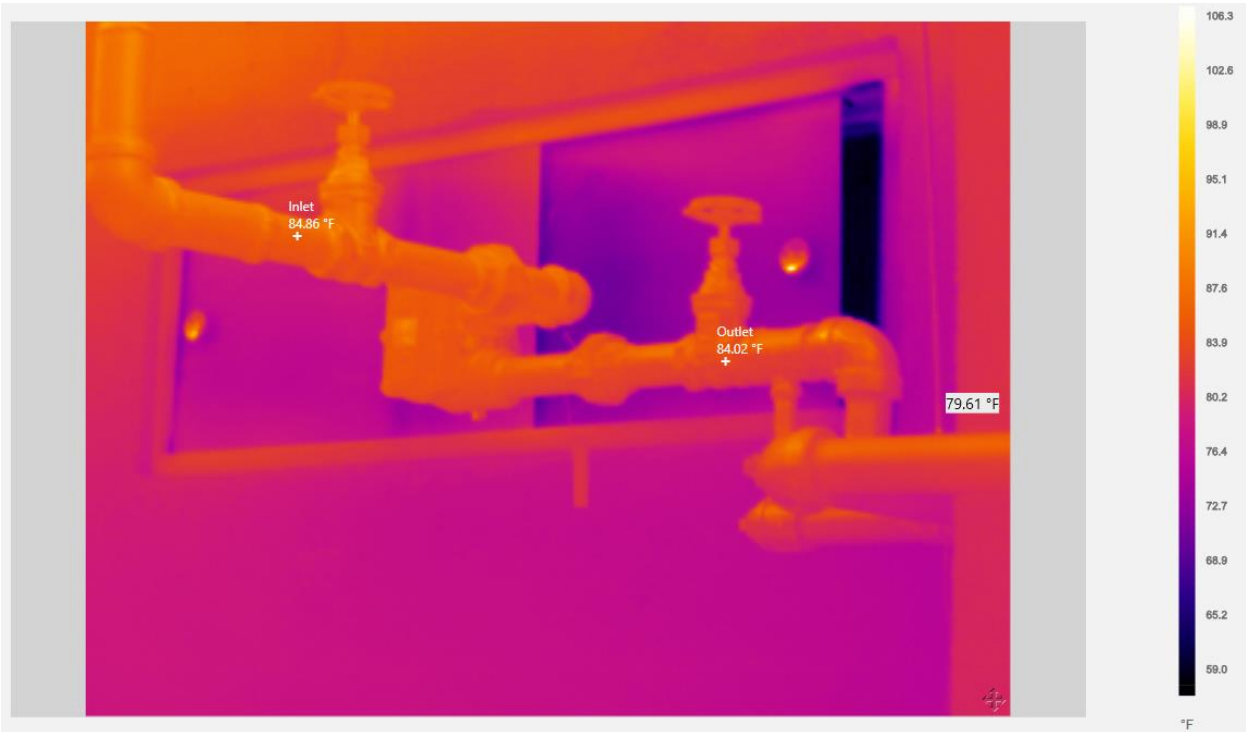
Building 2 Basement Trap C (not active)
