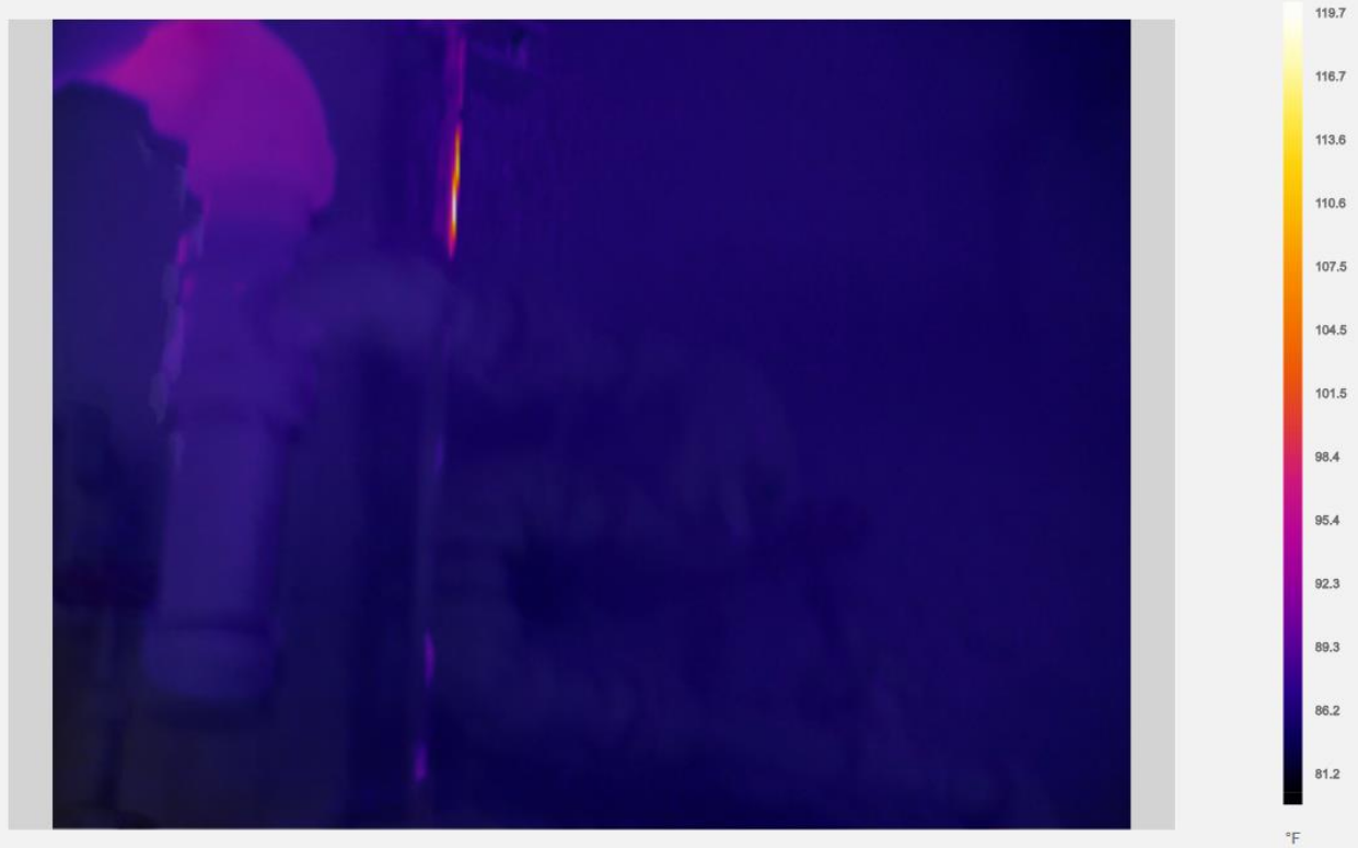
Building 3 Basement Trap C (not active)
