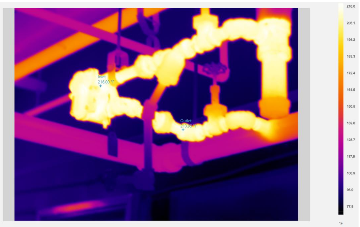
Building 6 Basement Trap A
