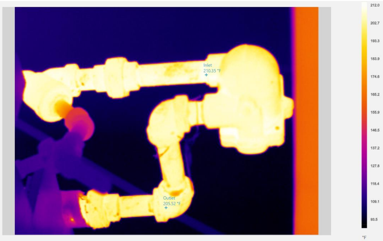
Building 4 Basement Trap A
